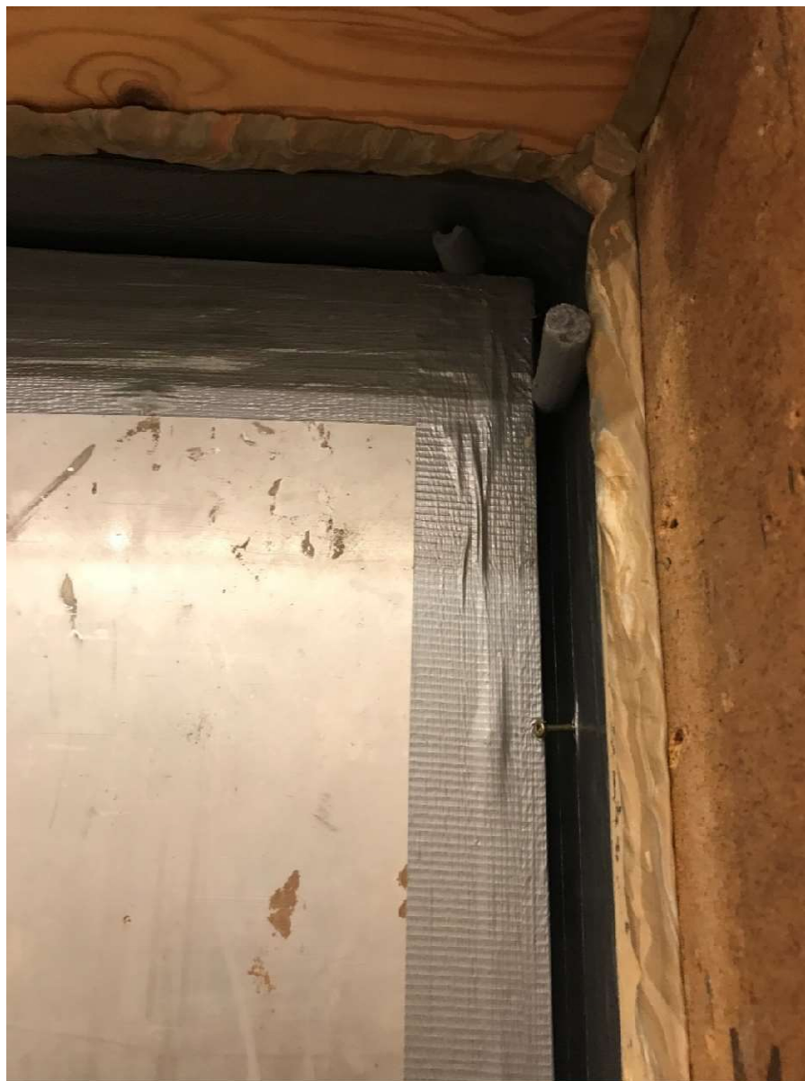
Figure 4: Picture of a part of the backing insulating rod (grey) used for controlling mortar depth on the receiving side (see Appendix 1). The slit is 15 mm wide.
